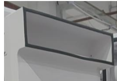
Air conditioning cold air outlet
